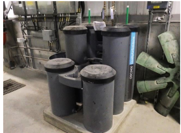
Photo 3.51 Fresh air rise (FAR) condensate separator
