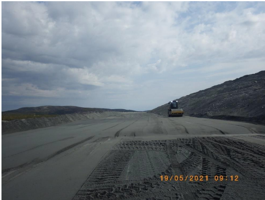
Photo 3.54 Deposition and compaction of processed kimberlite (coarse fraction) to raise a bearing downstream of the line centre
