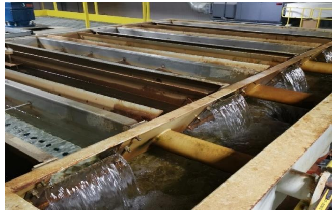
Photo 3.49 Treated water at the outlet of the lamellar clarifiers
