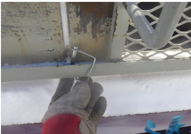
Photo 3.43 Safety latch – Dryhouse container
